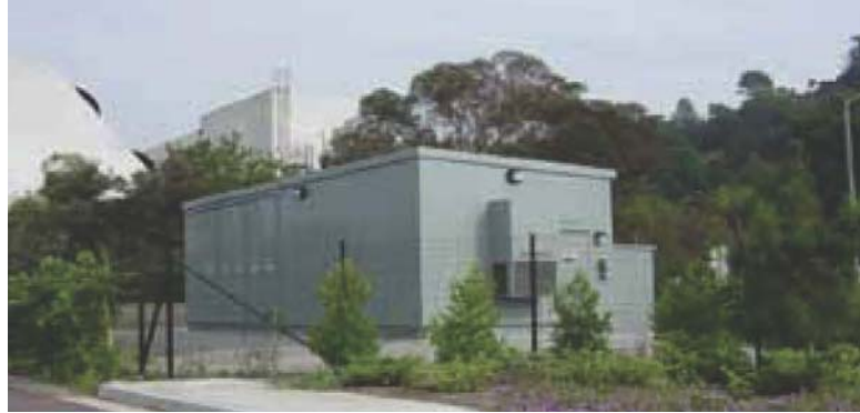
Figure 2: Example of a Traction Power Substation (TPSS)
